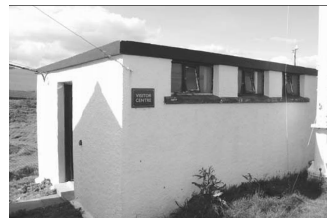
A view of the Visitor Centre showing seaward elevation where a large viewing window will be installed.
